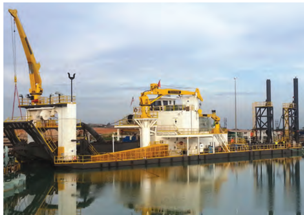
Dredge fully assembled and floating in the wet concentrator plant B mine pond at Moma.
